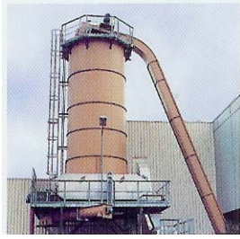
Wet sludge silo
